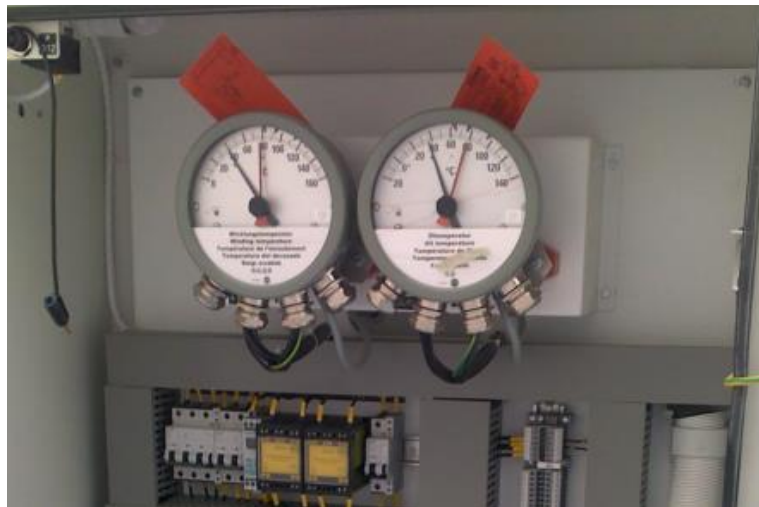
Figure 2. Gas density monitoring indicator
