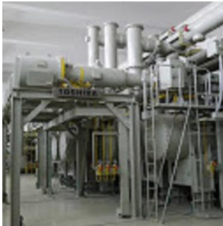
Figure 6. SF6 gas to air bushings
