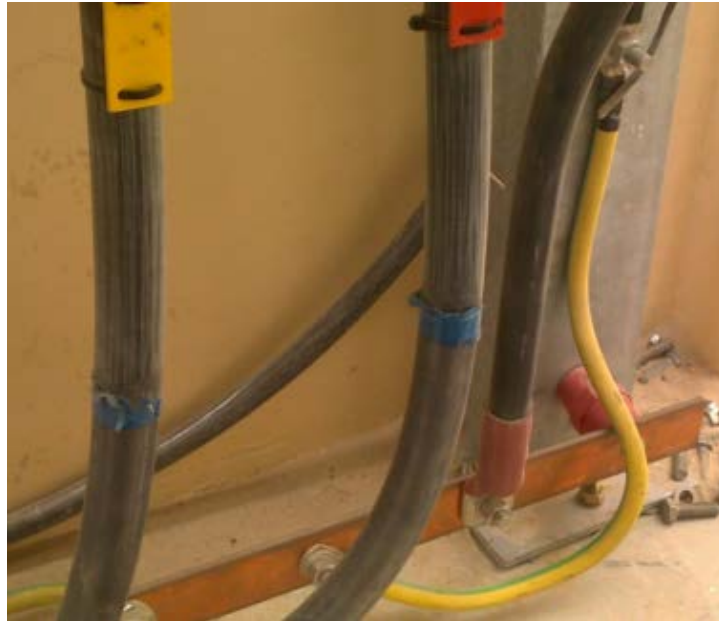
Figure 5. Ground/earth connection of GIS using bolts or a steel bar in the floor (a) Bolted GIS fixing with grounding connection (b) Steel bar is the floor including grounding connection
