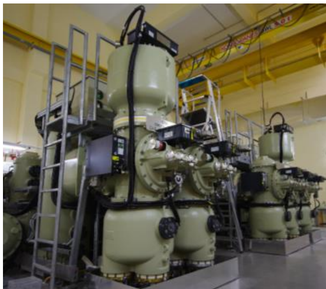
Figure 1. Ladders and platforms in GIS
