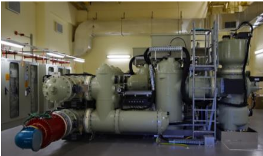
Figure 7. SF6 gas to cable connections
